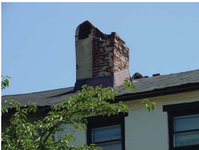
Example of chimney deterioration
