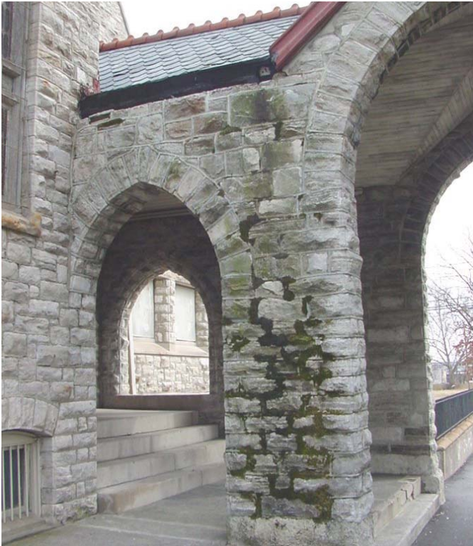
Damage caused by missing downspouts
