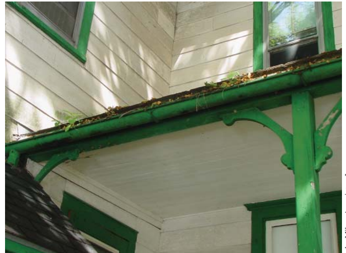
Gutters full of leaves and debris
